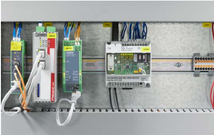
Figure 4: The individual system parts are segmented and protected by an upstream firewall — the FL mGuard security router from Phoenix Contact.
