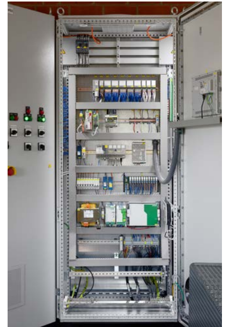
Figure 3: Along with the PLCnext Control device, other Phoenix Contact components, such as a security appliance, switch, and power supplies, are also installed in the rain overflow basin control cabinets.
