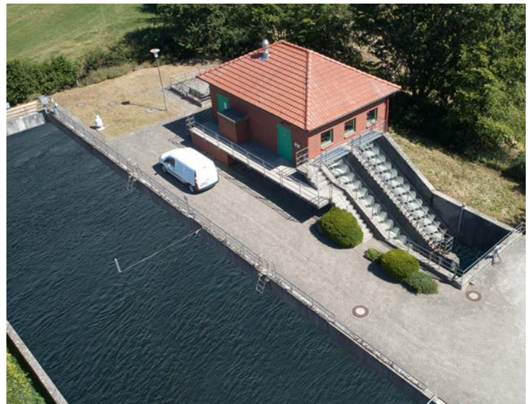
Figure 5: The rain overflow basin in Hoetmar has a volume of 1,000 cubic meters.
