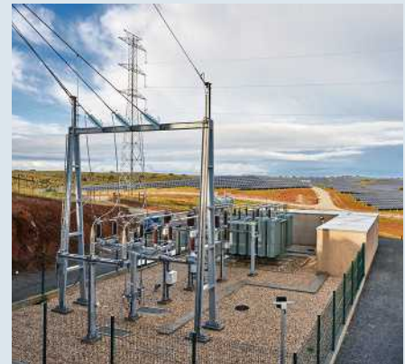
Grid connection with the feed-in controller from Phoenix Contact in a PV power station
