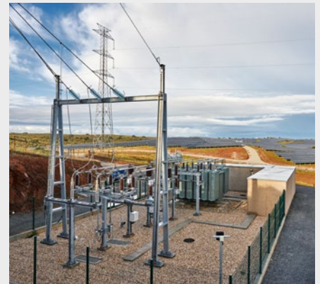
Grid connection with the feed-in controller in a PV power station
