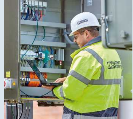
Use of the remote control and automation system in a power grid
