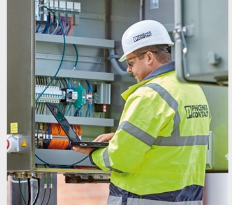
Use of the remote control and automation system in a power grid
