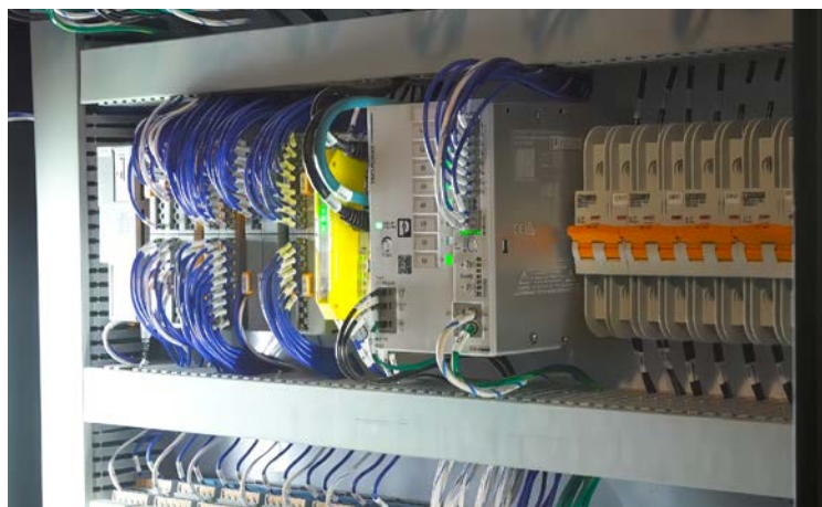
Figure 3: AHI Automation relies on numerous Phoenix Contact products, including TRIO power supplies with integrated circuit breakers, PLCnext Technology, HMI, and WLAN radios.
