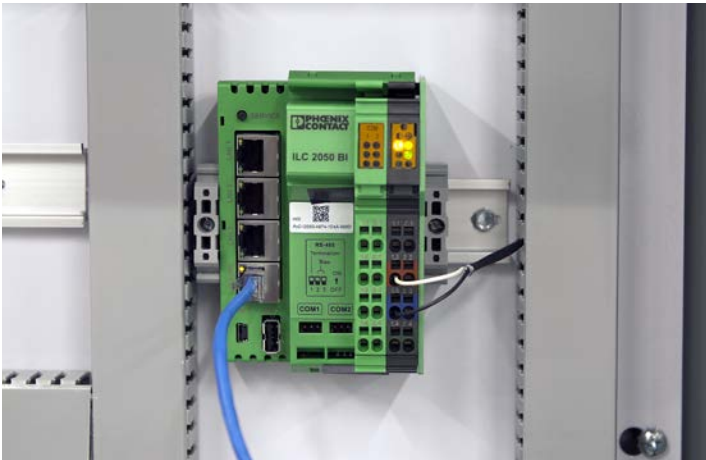
Figure 4: The Phoenix Contact ILC 2050 BI controller is the brain behind NOVVA’s cooling system. It ties all of the systems together and pulls in data from all kinds of devices, using Modbus, BACnet, and other protocols.
