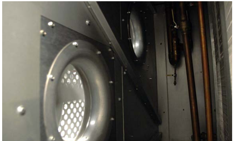
Figure 3: After the sealed glycol loop absorbs heat from the servers, massive air-cooled condensers push that heat into the atmosphere – without a single drop of water lost.
