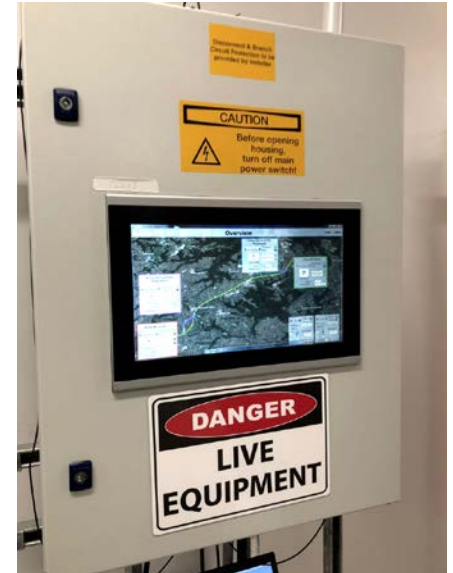
Figure 3: Control cabinet with the scalable control solution for configuring the complete tunnel lighting – and without programming effort. (Image source: John Ortika)
