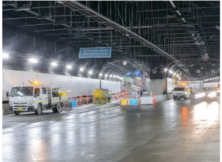
Figure 4: Schröder and Phoenix Contact technical experts from Belgium and Germany supported the commissioning despite COVID-19 travel restrictions, as the ATS control system allows remote access via modem. (Image source: Transurban/NorthConnex)
