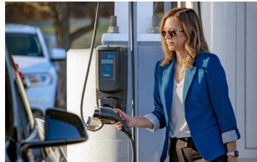
EV charging stations for employees and visitors
