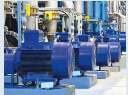
Motors and pumps in an industrial facility
