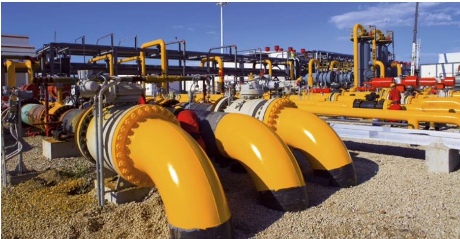
Fig. 96: Typical application field: gas compression station
