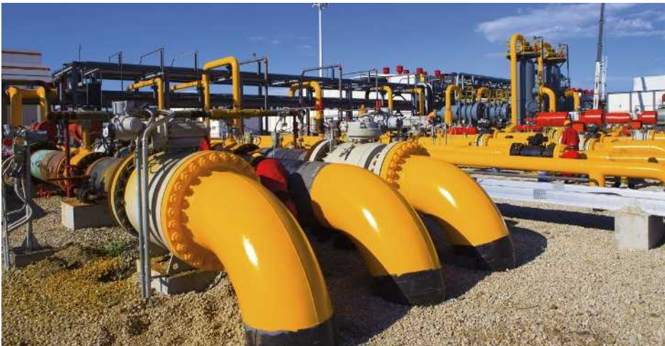
Fig. 96: Typical application field: gas compression station
