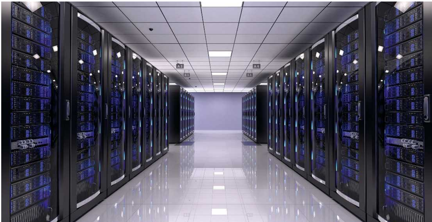
Fig. 68: Data center with a DC power supply system with linear source characteristics
