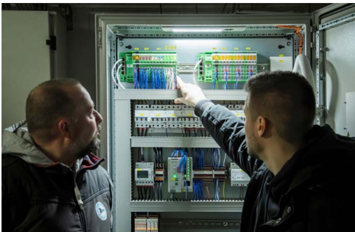
Figure 2: Pumps are controlled using the open ILC 2050 BI building controller.
