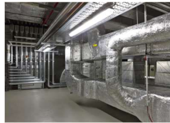
HVAC Heating, ventilation, air conditioning
