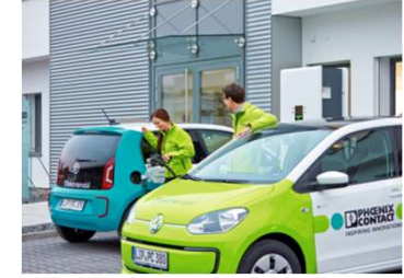
Exterior lighting with integrated E-Mobility charging station
