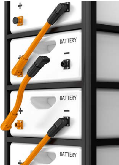
Figure 7: Battery pole connectors and cables
