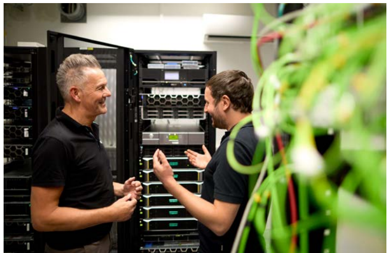
Figure 3: Close cooperation with the IT department has enabled well-organized interfaces and responsibilities.
