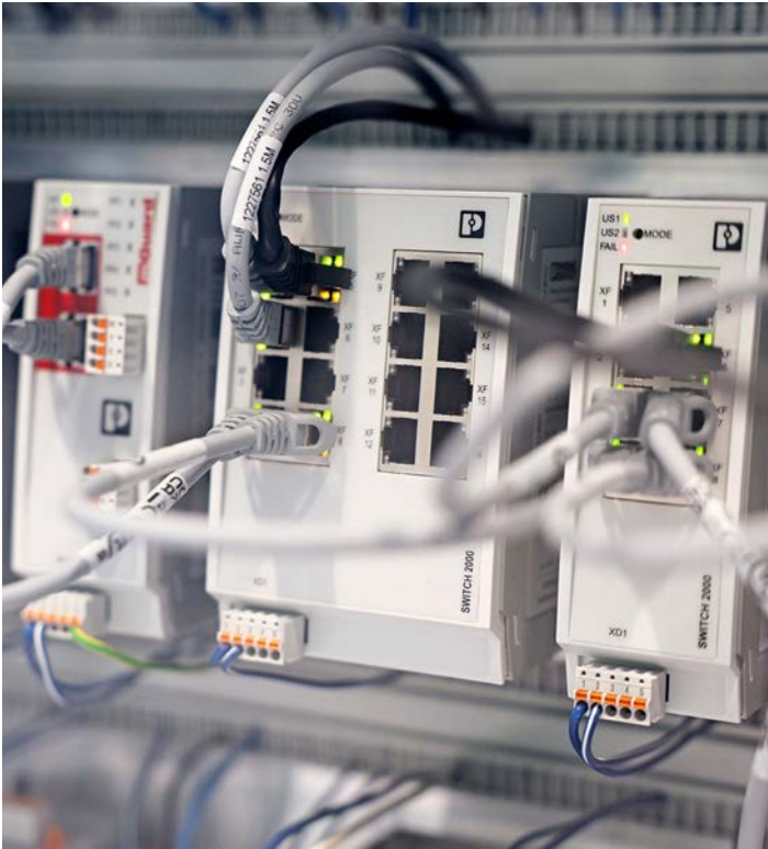
Figure 2: Use of managed switches and security routers in the control cabinet.
