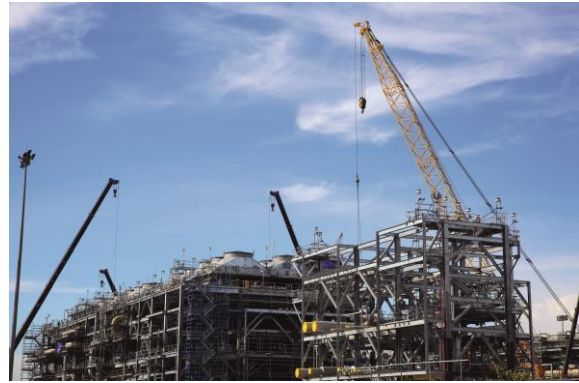
Figure 1 - Modularisation provides increased transparency to system operators so that they can dedicate greater attention to the use of their own system (image source: Shutterstock)
