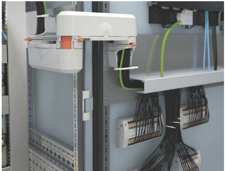
Safe conductor routing to the FAME test disconnect system in the control cabinet door
