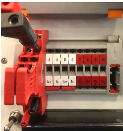
Figure 6: Two-pole test probe safely shorts CT and isolates it from the circuit.
