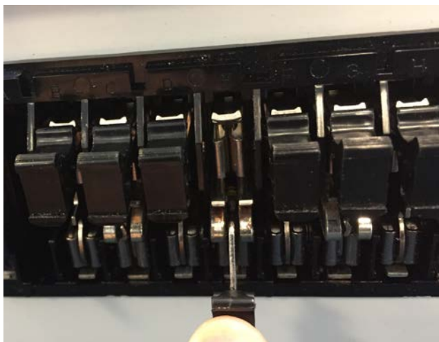
Figure 1: Opening knife switch to expose test point.
