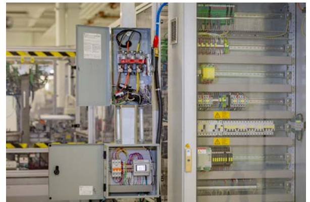
Figure 1: Like many manufacturers, Phoenix Contact is looking for ways to improve energy efficiency in its manufacturing process.
