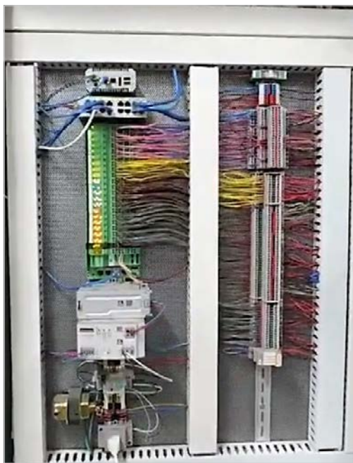
Figure 4: Phoenix Contact's industrial-grade control and I/O hardware form the backbone of the building automation system.
