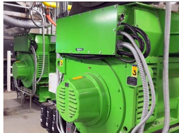
Figure 3: The cogeneration plant burns fuel to create electricity.
