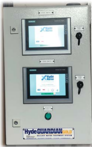
Figure 4: Operator interface terminals (OIT) displays or human machine interfaces (HMI) on the Hyde Guardian BWMS are connected to the mGuard, so that the crew members in the barge control house can see what the systems are doing.
