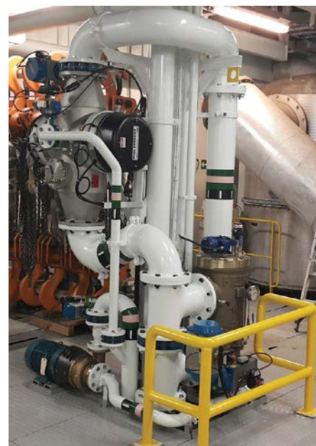
Figure 1: Ballast systems are installed deep in the hull of the vessel. The Faraday Effect makes it difficult for electromagnetic fields to penetrate in this area, so cellular communication is not always possible.
