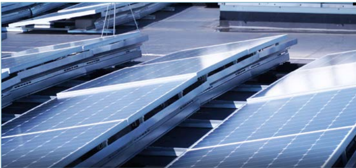
Figure 3: The solar installation will help Phoenix Contact meet its long-term corporate goal of becoming a carbon-neutral company.
