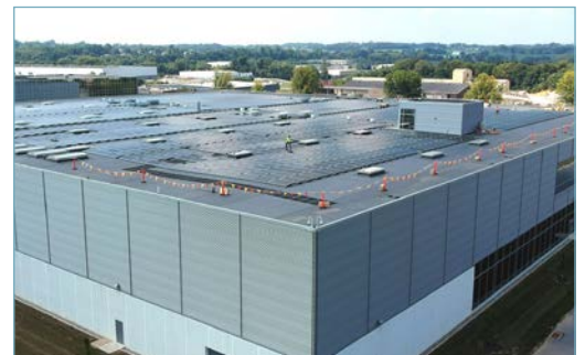
Figure 1: Phoenix Contact installed a nearly 1-megawatt photovoltaic system on the roof of its logistics center.
