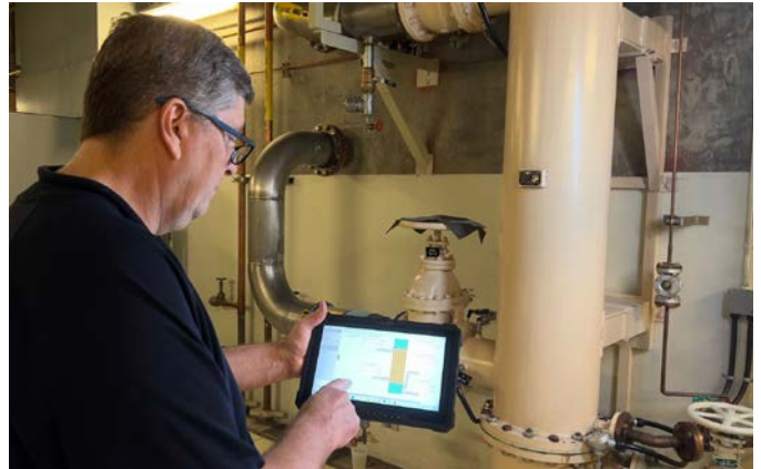
Figure 3: The technicians now have access to real-time SCADA data right on the plant floor, so they can take action on alarm situations much more quickly.
