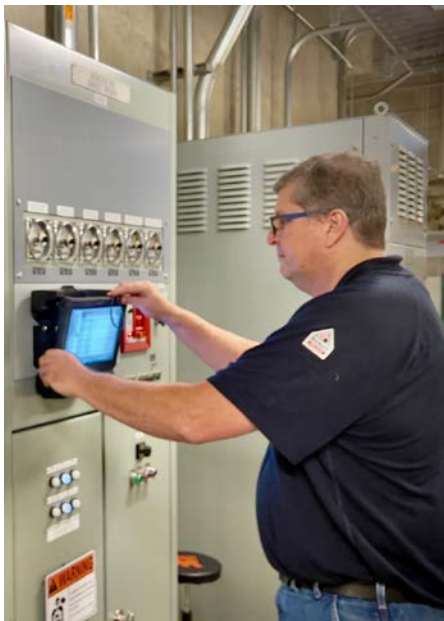
Figure 2: Derek Stone uses the Dell Latitude Ruggedized Tablet to monitor conditions on the plant floor.
