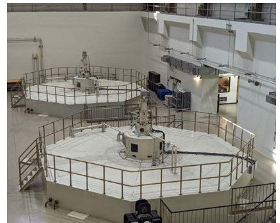
Figure 1: The Lucky Peak Power Plant can generate up to 101 megawatts of electricity.
