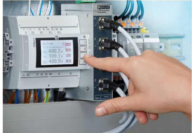
Electrical energy measurement
