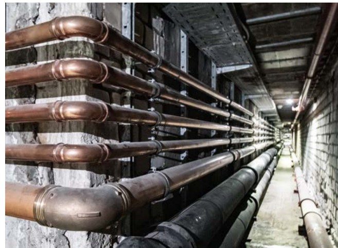
Underneath the plant site, there is an underground world with miles of supply lines
