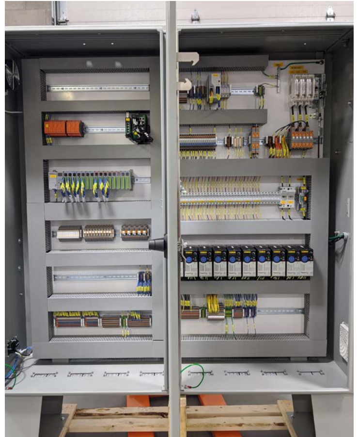
Figure 4: Novum condensed the control system into just two standing cabinets, compared with three or four in the original system.
