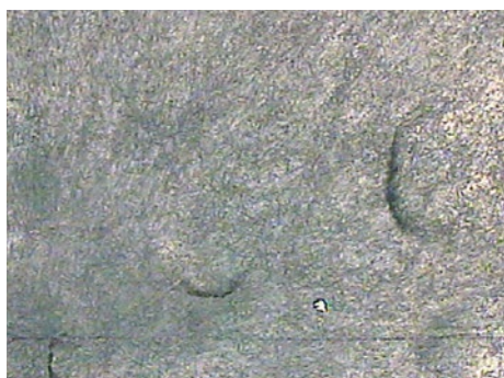
Fig. 29: Failed level – blister formation
