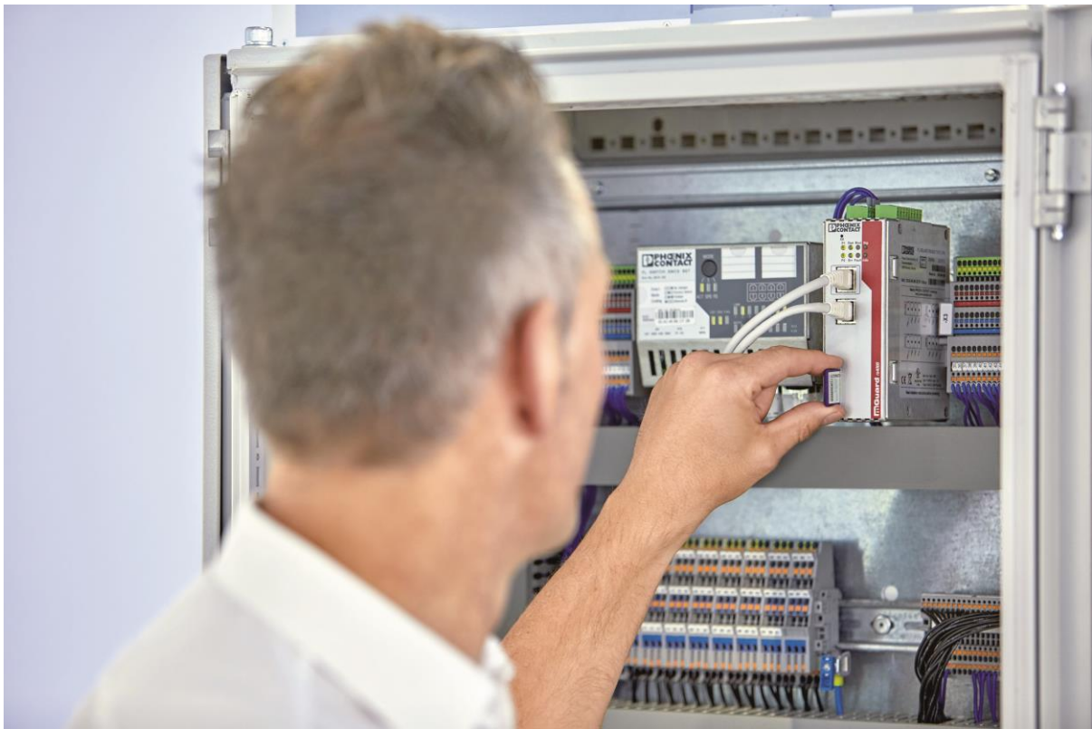
Figure 4 - Phoenix Contact provides a wide range of services in the security environment
