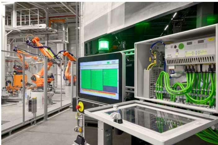
Figure 5: Industrial PCs from Phoenix Contact are installed as main and secondary control consoles on a pedestal.
