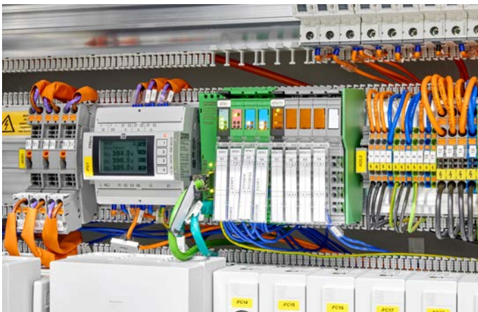
Figure 2: The multifunctional EEM-MA 370 measuring device records energy consumption data.
