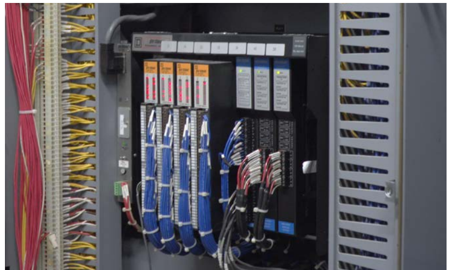
Figure 1: The old PLC, installed in the 1990s, was in danger of failure, which could have disastrous consequences for the residents who rely on the water supply.
