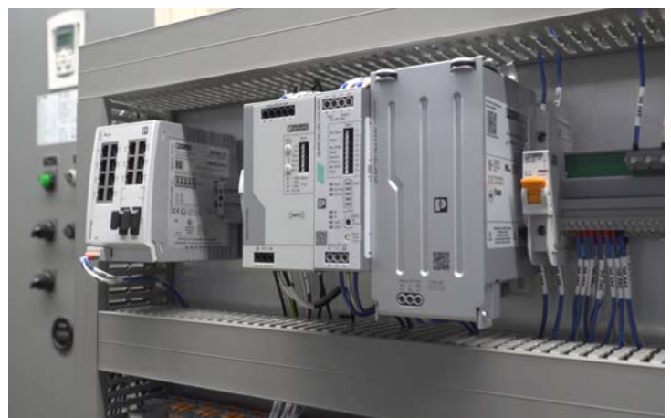
Figure 3: Each station on the ring has a DC UPS battery backup for power redundancy. This further increases the system’s reliability and resilience.
