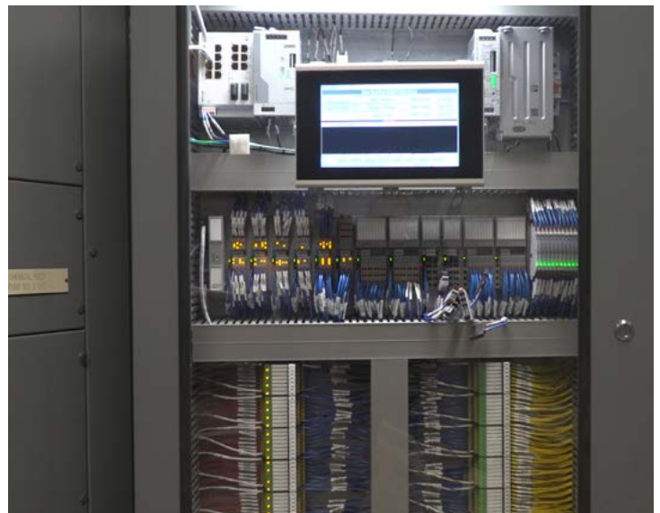
Figure 5: With the new modern control panel, the Industrial Internet of Things (IIoT) holds the promise of enhanced asset management and process efficiencies by gathering and analyzing data from a wide range of industrial devices. Artificial intelligence and machine learning will augment applications such as predictive maintenance and energy management.
