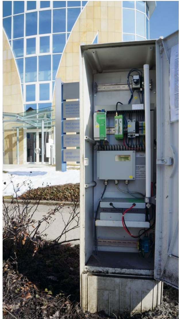
Measuring station for recording the amount of heat at the Albstadt-Sigmaringen University of Applied Sciences
