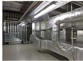
HVAC Heating, ventilation, air conditioning
