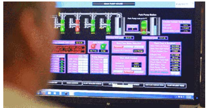
DYNAC software makes it easy to monitor and control pumps around the facility, and operators can view all system conditions at any given time through the HMI in the main pump house.
