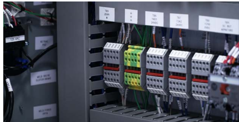
Figure 4: NSRW uses a variety of Phoenix Contact terminal blocks and fuse holders, including the QUATTRO series.
